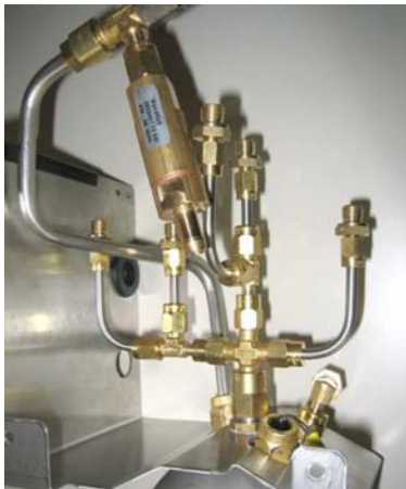
Boiler subassembly pre-fabricated by SERTO, mounted and installed by customer
